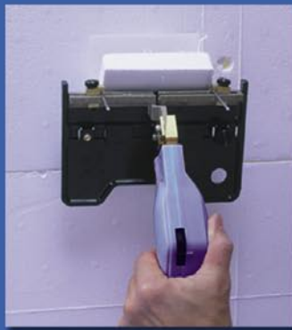
Use the QC Hot Knife with the Groove Sled attachment and electrical box blade to make the cut
