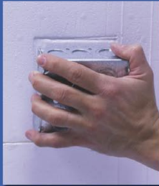
Use the electrical box to create an outline on the foam wall
